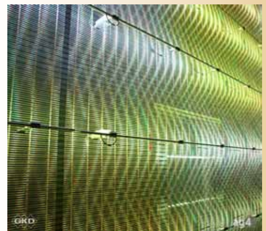
The stainless steel mesh surface of this Illumes® installation in Torce, France, shines with reflected sunlight during the day and glows with an ever-changing display of light and color at night.
